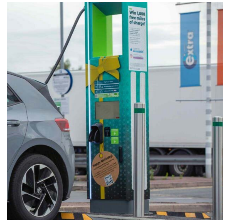
Figure 17. EV charging 'Super Hub' at Moto Thurrock (credit: Gridserve)
